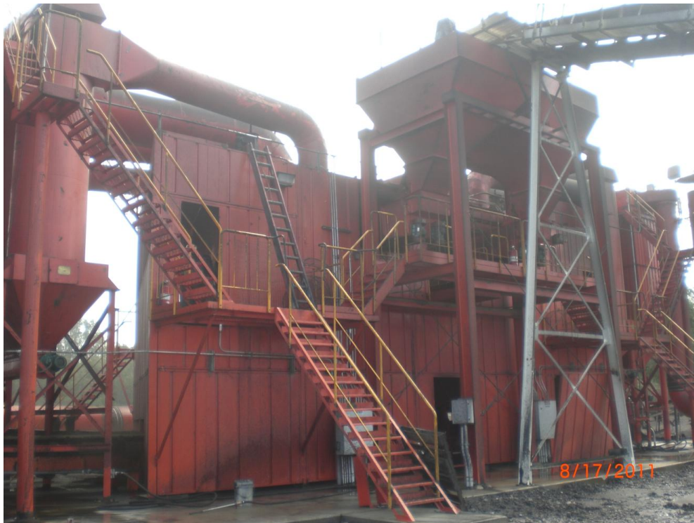
Figure 14: First commercial installation of the FGX Dry Separator in Illinois by the Eagle River Coal Company.
