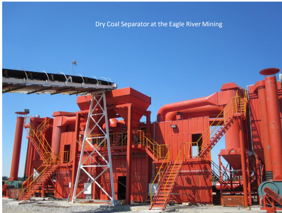
Figure 5. FGX-24A in operation at the Eagle River Mining
